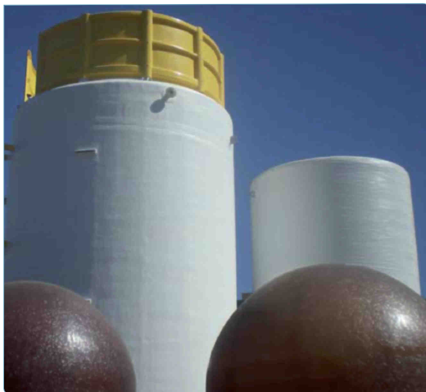
Fig.5 :An example of a sodium hydrochloride FRP tank
