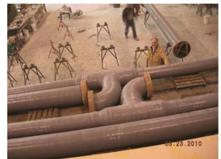
Figure 4 FRP pipe used in National 9/11 Memorial Fountains at New York City's World Trade Center
