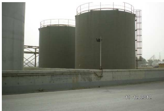
Figure 1 1500 m 3 C-PVC+ FRP Storage Tanks installed at a Saudi Arabia site
